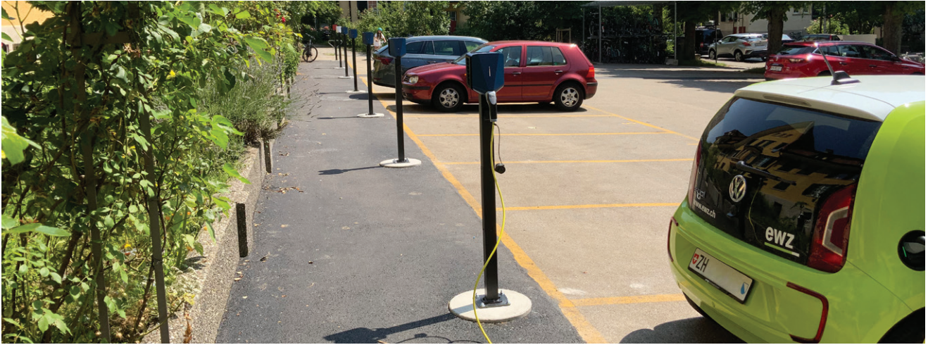
Parkings Stolzstrasse 30, Zurich (source: ewz)
